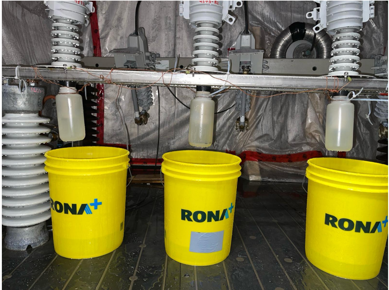
Figure 5 –Detail of the oil containers for the bushings
